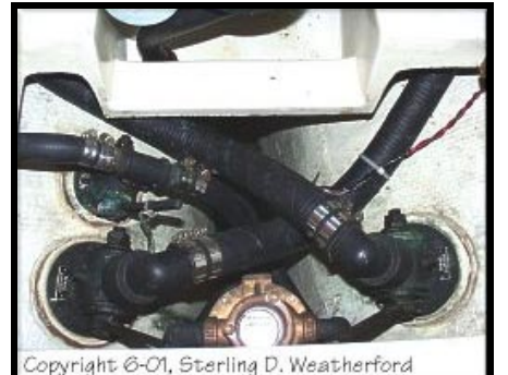
Copyright 6-01, Sterling D. Weatherford
