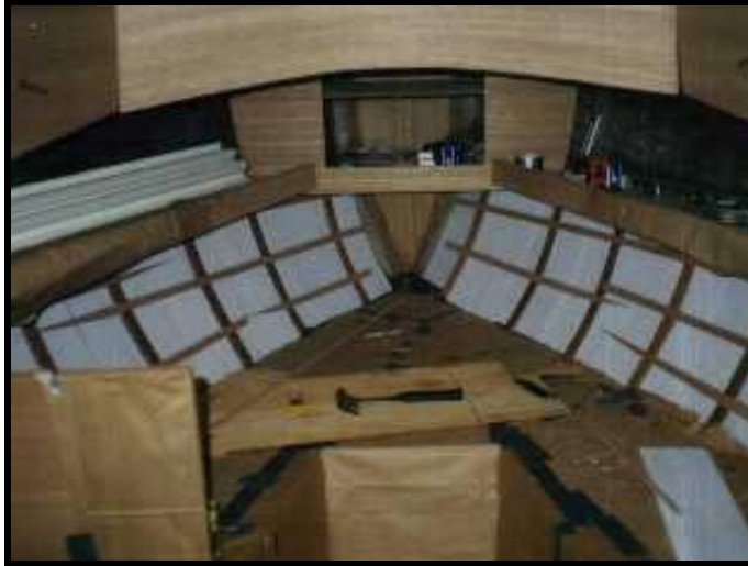
Forward Cabin Insulation – A small shelf was added on both sides of the forward cabin. Notice the frames in place for the ceiling, the roughed-in forepeak locker and the insulation along the hull.
