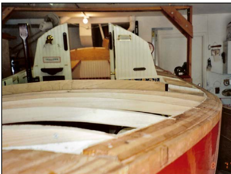
Next, full beams were added to match the camber. Photo: Bob Collier © 2015
