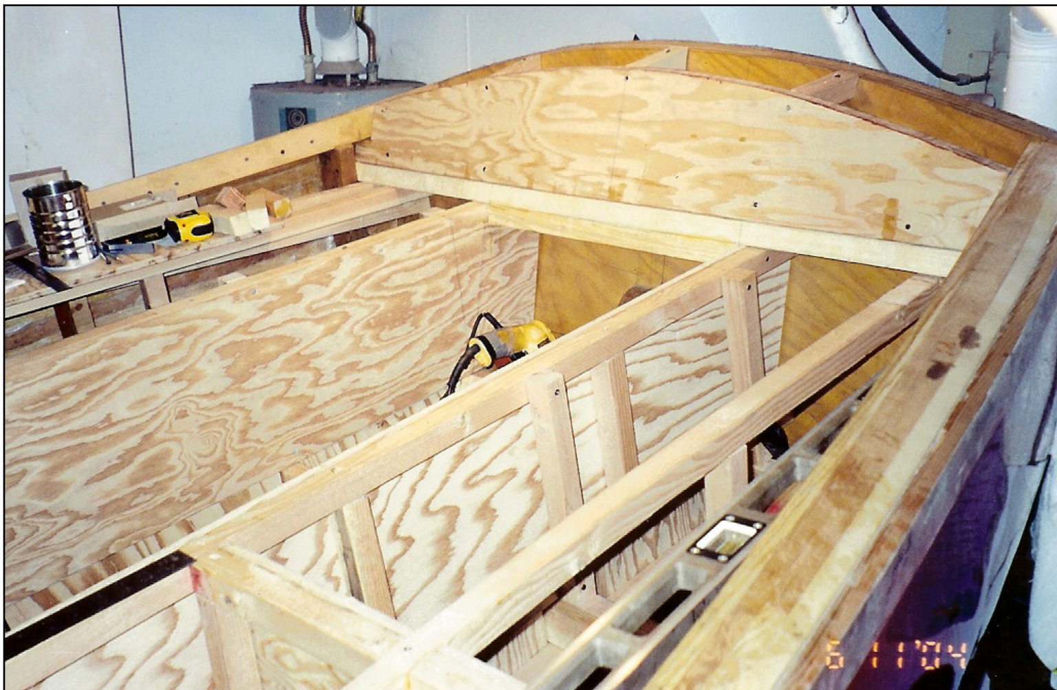
Adding the panels to the cockpit of s/y RED RASCAL . The cockpit is beginning to take shape. Photo: Bob Collier © 2015
