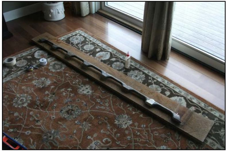
Using the old rails as templates on the new teak board. Photo: Randy Richardson© 2014
