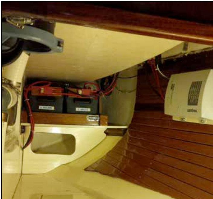
The new battery shelf, charger, and fresh wiring. Photo: Ian Williams © 2013
