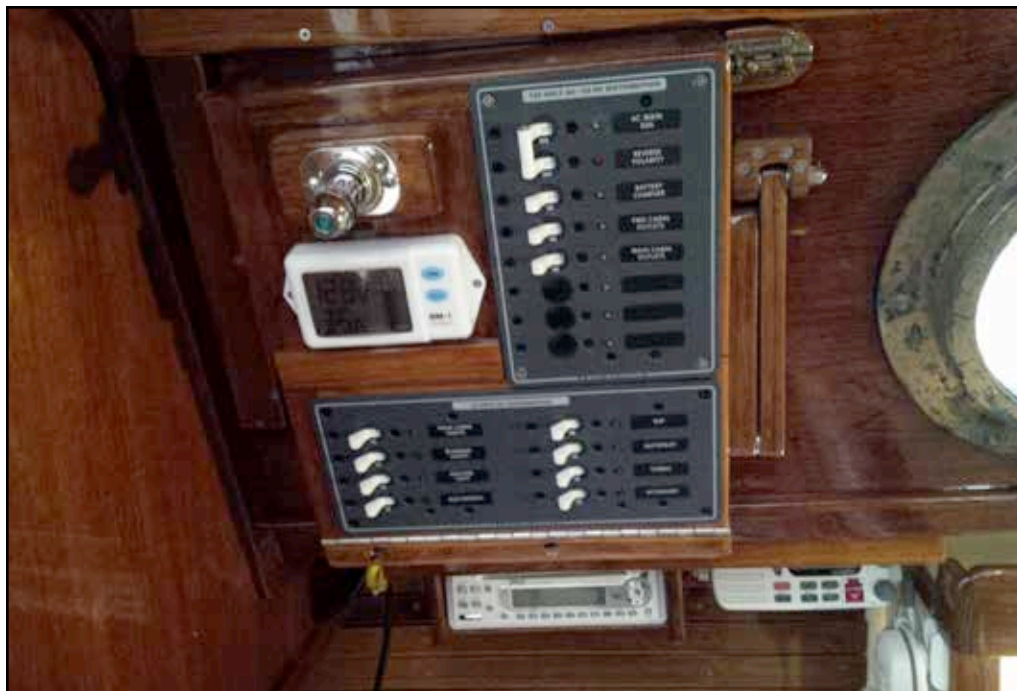
A custom AC and DC electrical panel was built complete with a support hinge.
