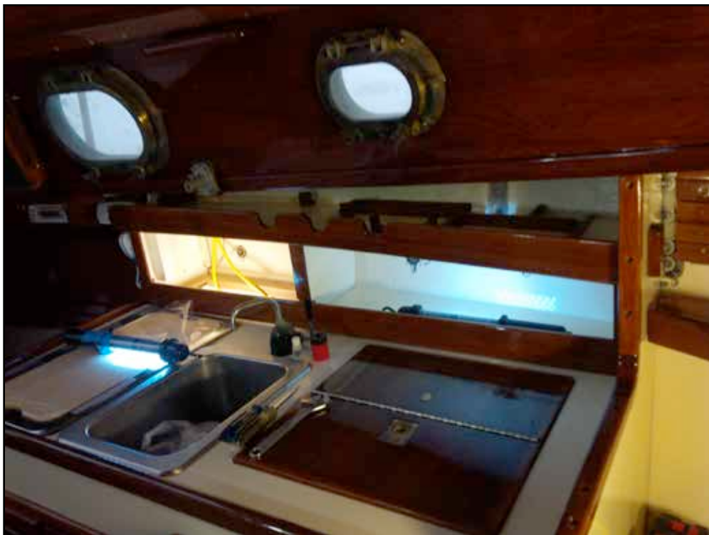
The galley was rebuilt with a new storage area. Photo: Ian Williams © 2013
