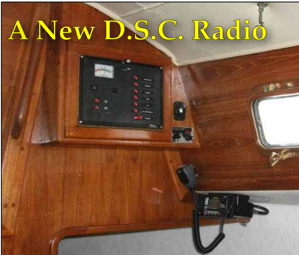
My new West Marine D.S.C. V.H.F. Marine radio installed above the quarterberth. Photo: Randy Richardson © 2013
