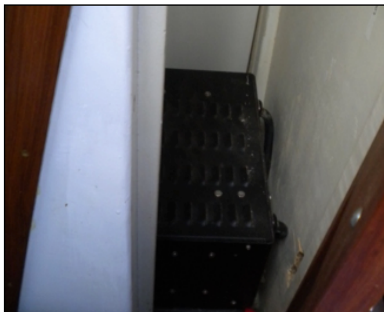
Power supply shown in closet, before woodwork. Photo: Bill Cartwright © 2013
