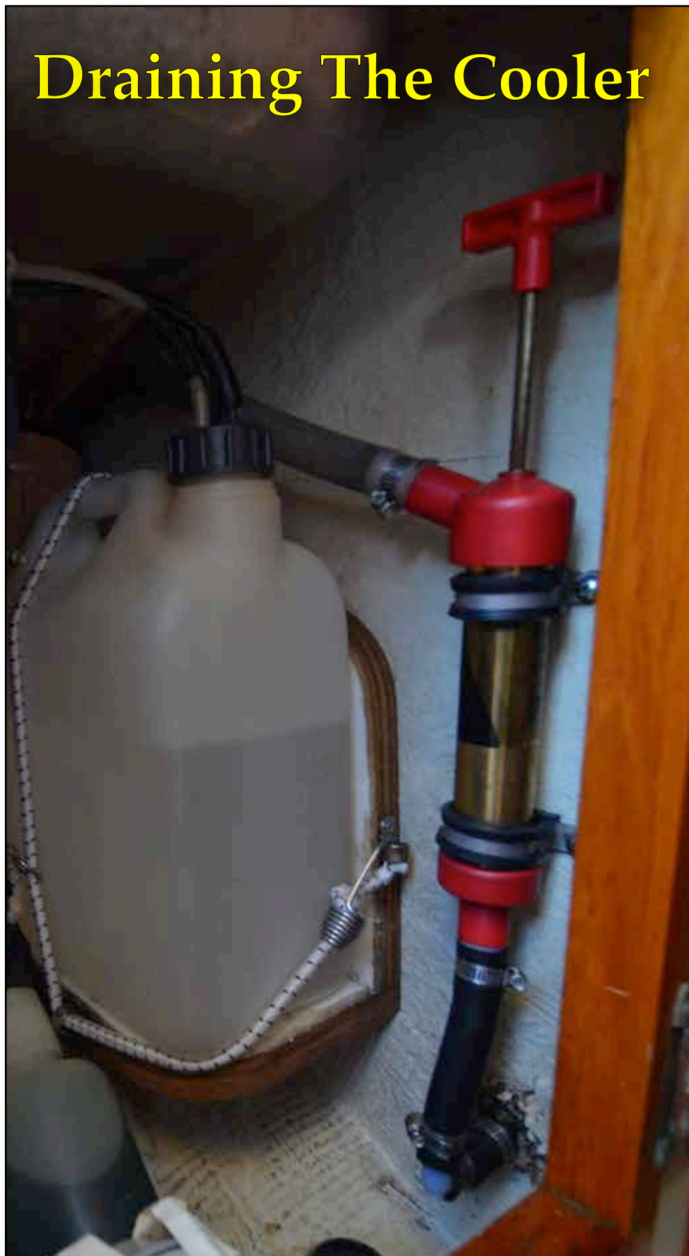
Rather than draining into the bilge, a pump is used aboard s/y KIRI . Photo: Tom Davison © 2013
