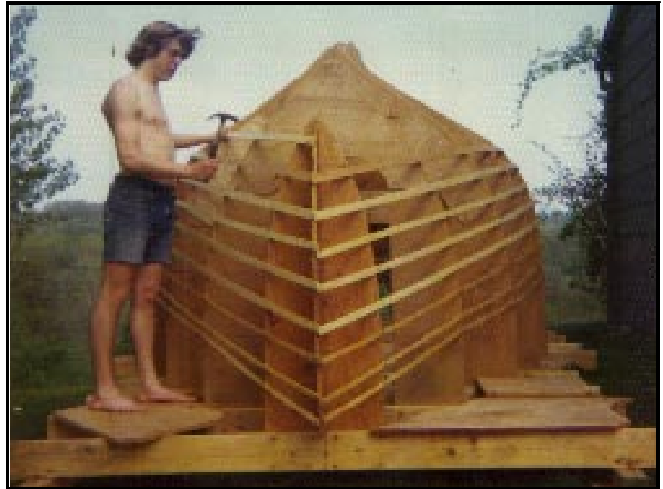
Attaching the lathe to the mold frames - the QED begins to take shape, but there is still a long way to go to complete the mold (let alone the boat).
