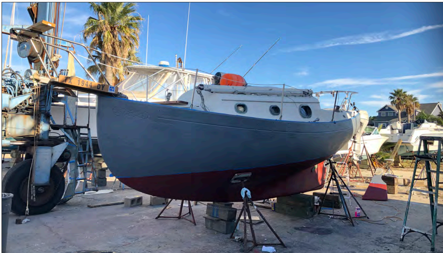
Two primer coats were applied to the topside of the hull. Photo: Jamie White © 2020
