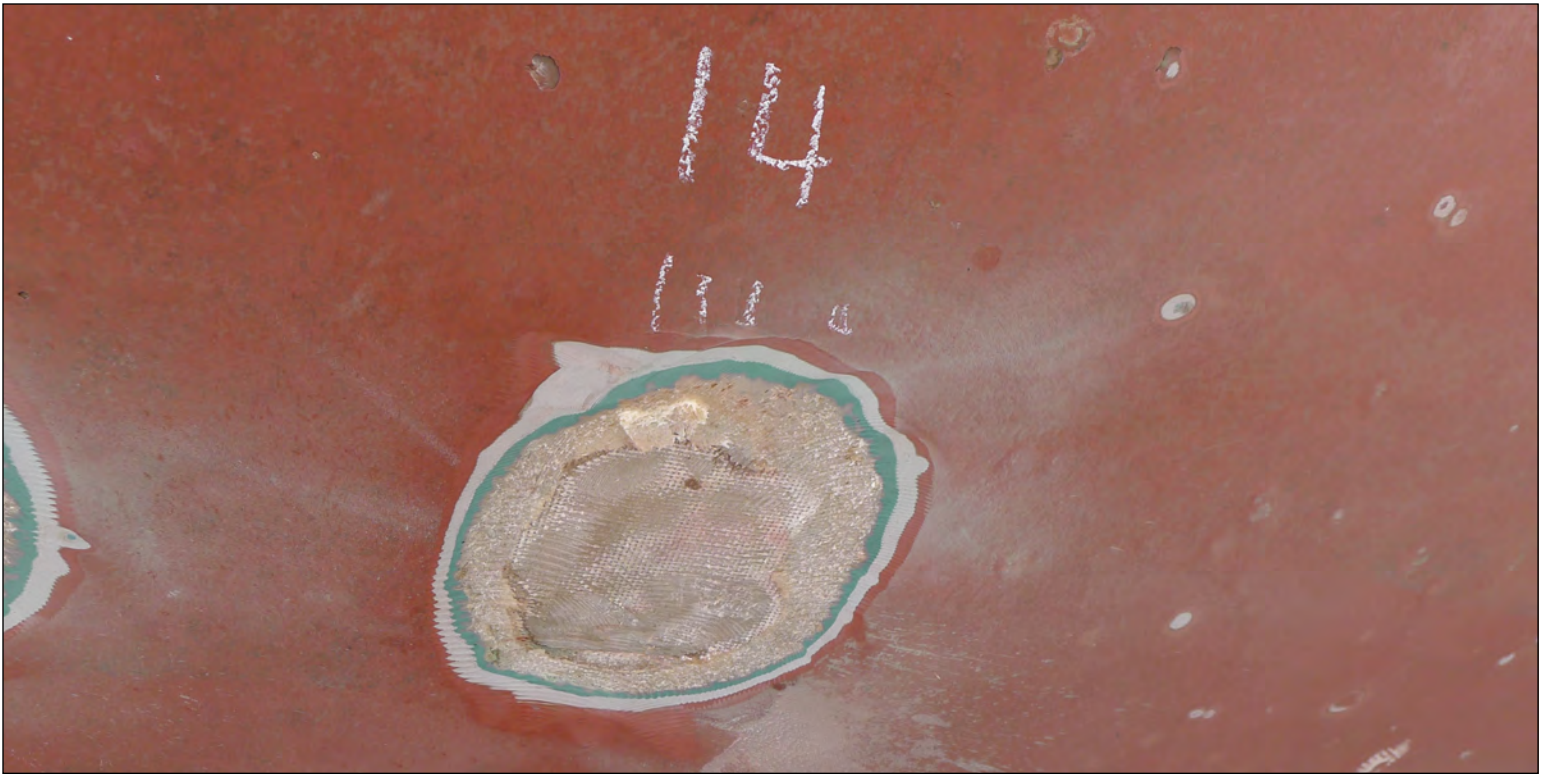
Blister #14 grinding almost completed. Note the different layers and that the blister did not extend into the structural roving. Photo: Jamie White © 2020
