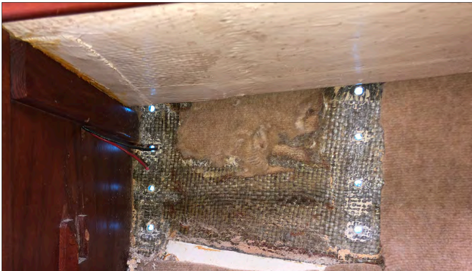
After cleaning up the faying surfaces of the hull liner to obtain a good watertight seal under the backing plate. Note the thick heavy fiberglass roving our Flickas were laid up with by Pacific Seacraft. Stout! Photo: Jamie White © 2020
