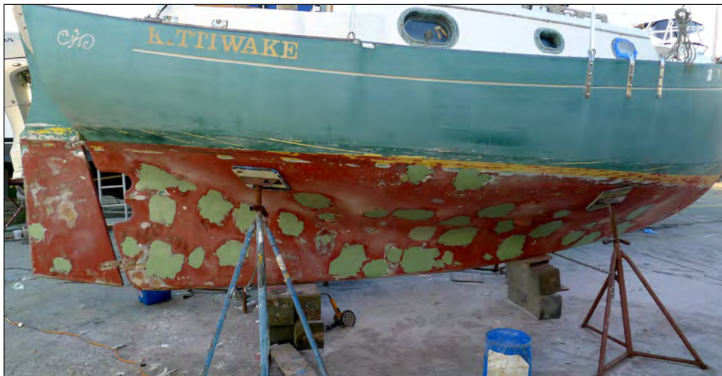
Two-part marine grade epoxy filler was applied over the repairs. Photo: Jamie White © 2020
