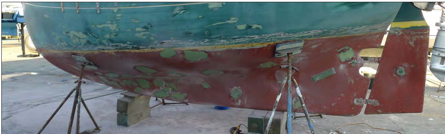
Others in the yard were improperly using automotive filler that will absorb water. Photo: Jamie White © 2020
