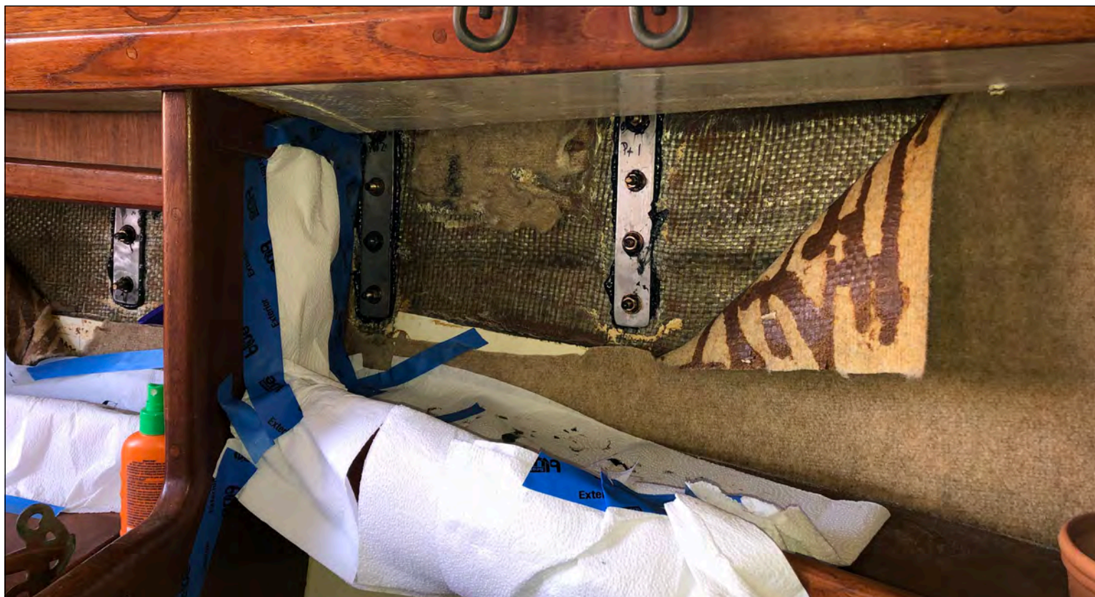
Portside backing plates installed and bedded with 3M 4000 polyurethane sealant. Photo: Jamie White © 2020
