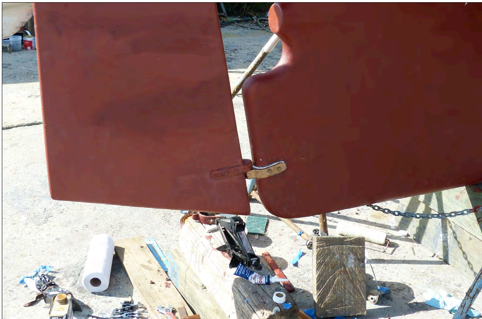
Completed replacement of the lower gudgeon of s/y DULCINEA . Photo: Jamie White © 2020
