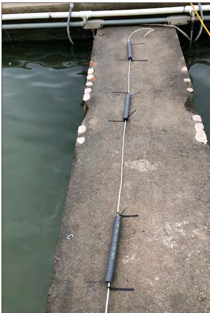
VHF antennae cable with foam noodles and cable ties ready to be passed through the mast. Photo: Jamie White © 2020
