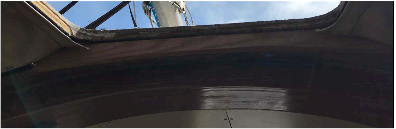
While I was at it I added a small arch to the hatch cutout frame just because I could. Fortunately the plywood deck was not damaged or wet. Photo: Jack Russell © 2020
