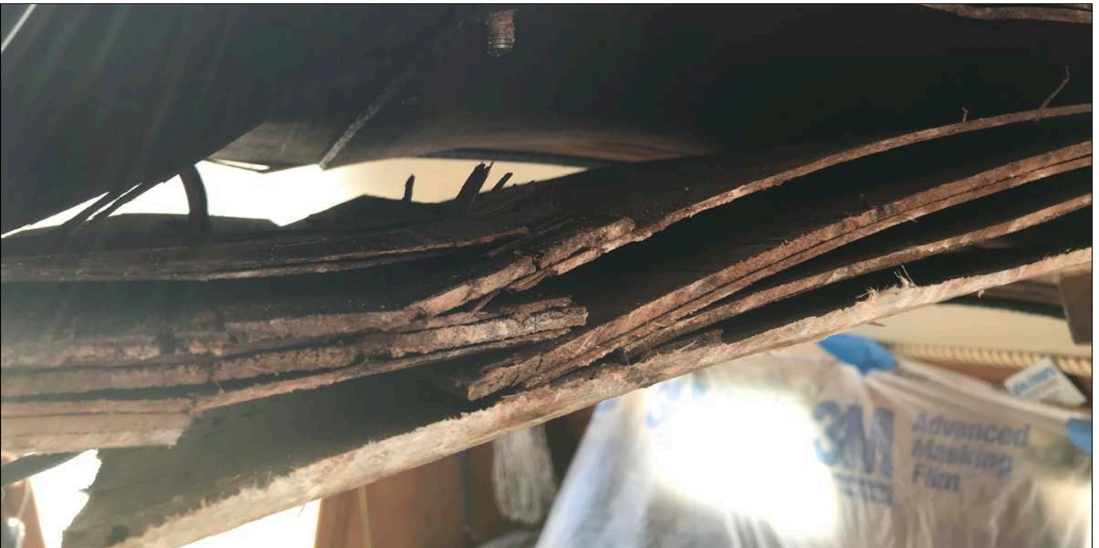
Next, took a cut-off wheel to the outside fiberglass encasement and here is what I found. The wood was actually dripping with water. No surprise really. Photo: Jack Russell © 2020
