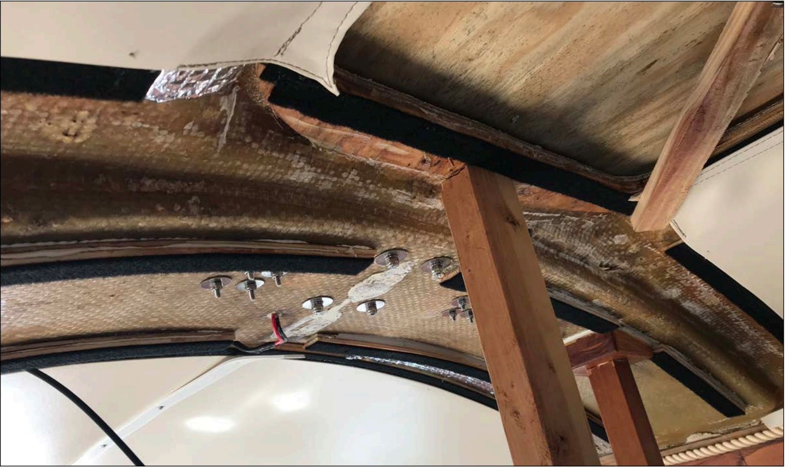
Here is what that glassed-in arch looks like with a temporary 2x3 on a scissor jack to hold it back in place. Photo: Jack Russell © 2020
