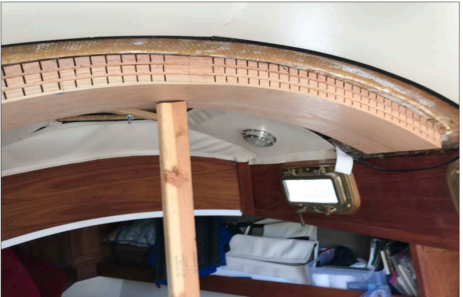
The next step was to cut the ends at the perfect angle to match those end blocks mentioned earlier. A scary procedure since you only get one chance! Then jack the unit into place and glue it to the roof. Photo: Jack Russell © 2020
